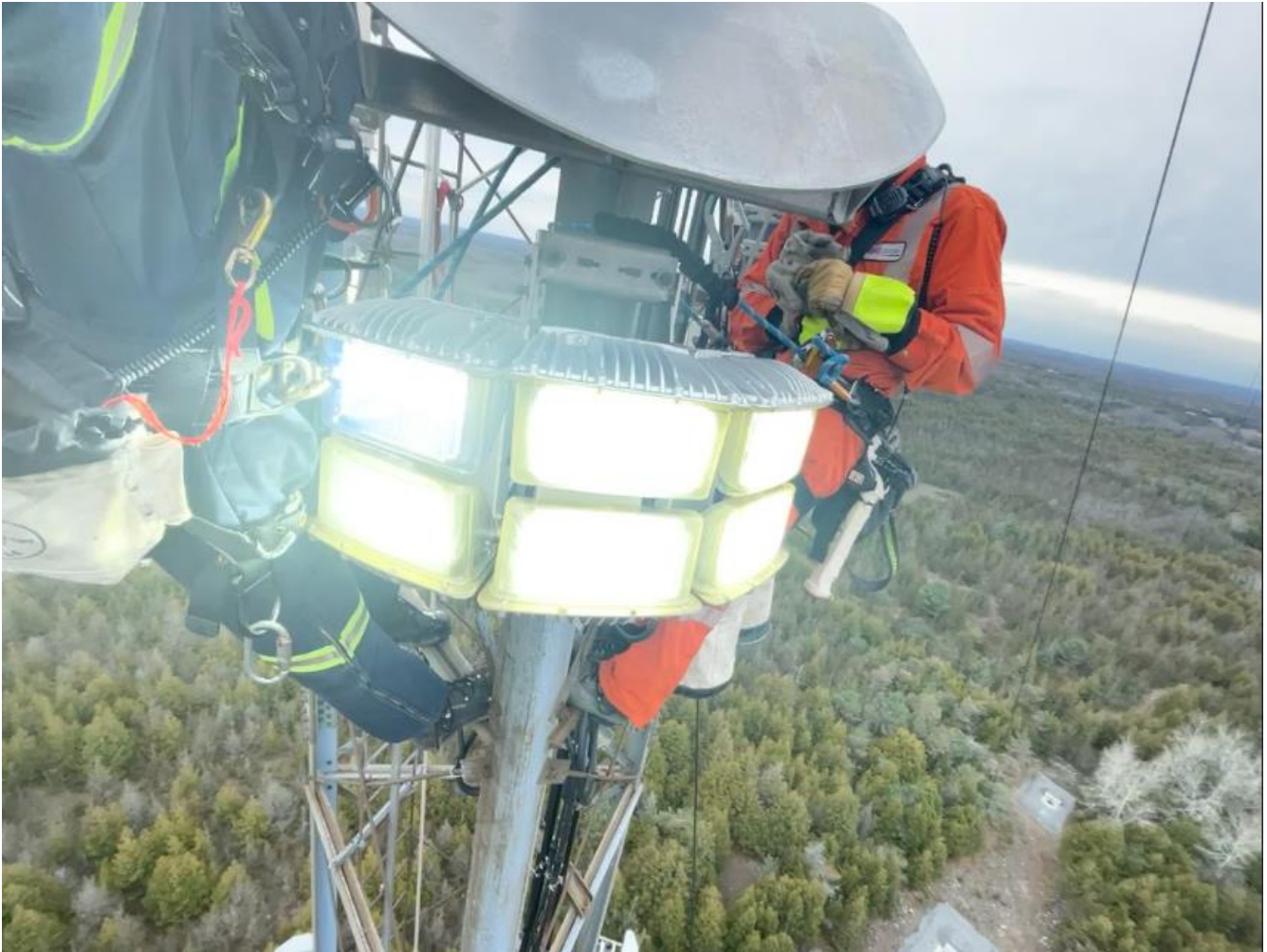
Belleville ON Technostrobe LED Lighting system
