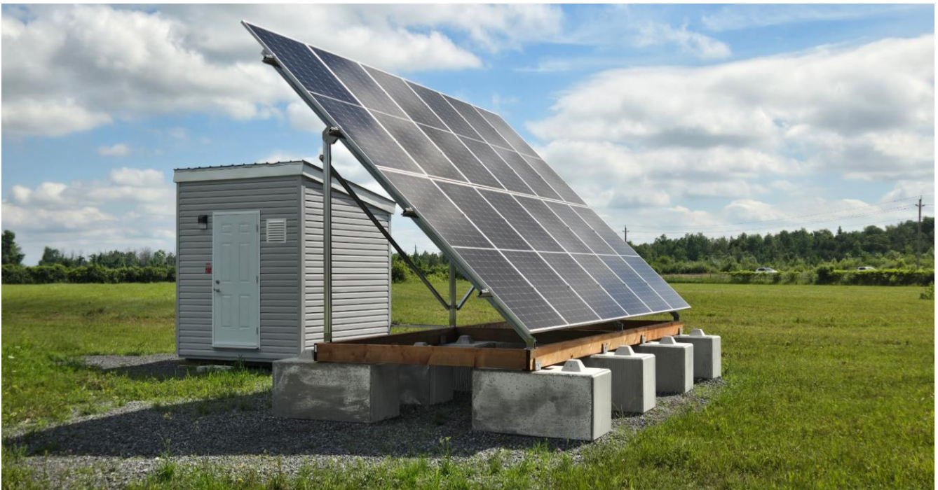
Solar panels being tested at the Innovation Hub in Carp, ON
