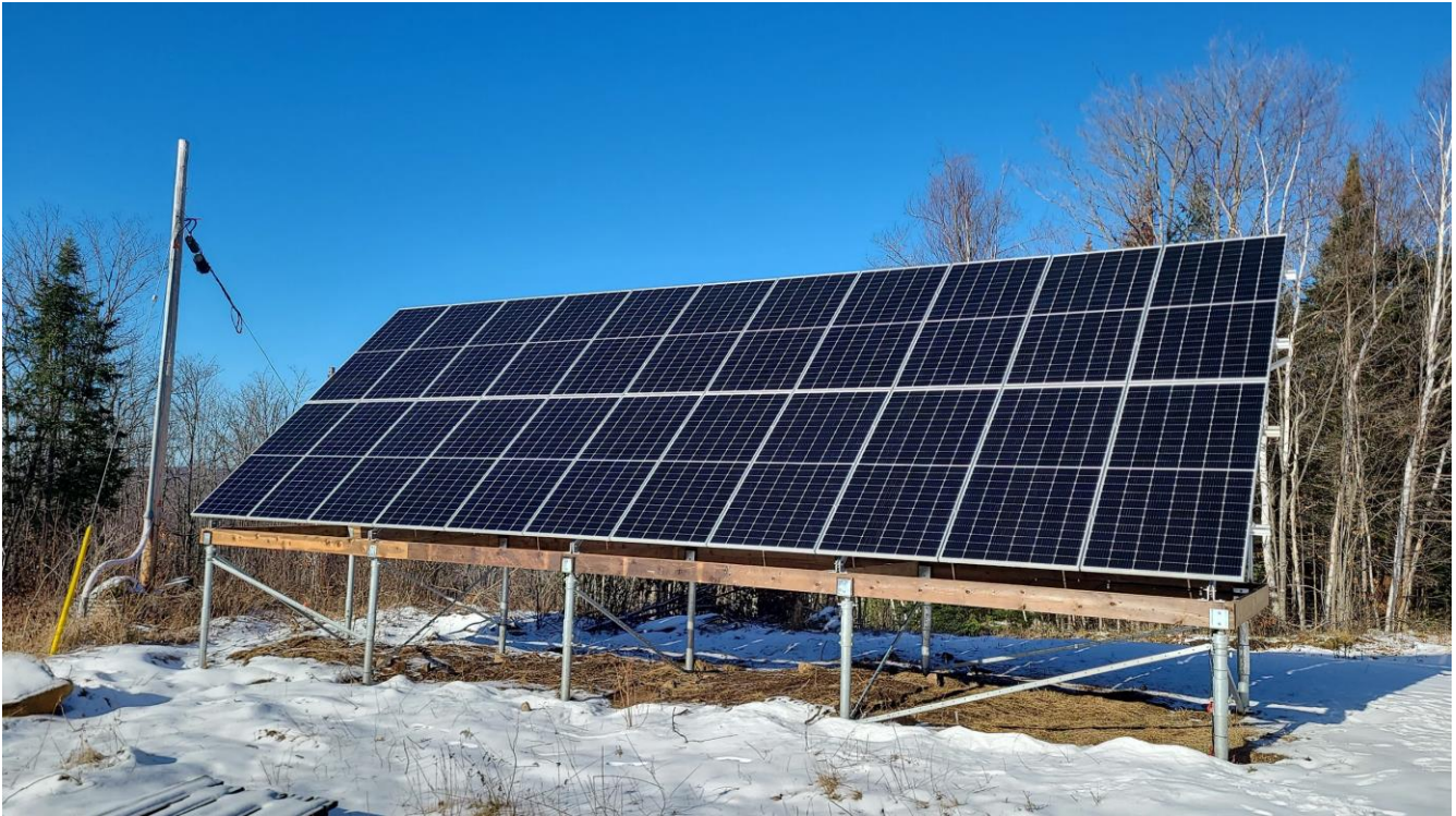
Solar panels in Whitney, Ontario
