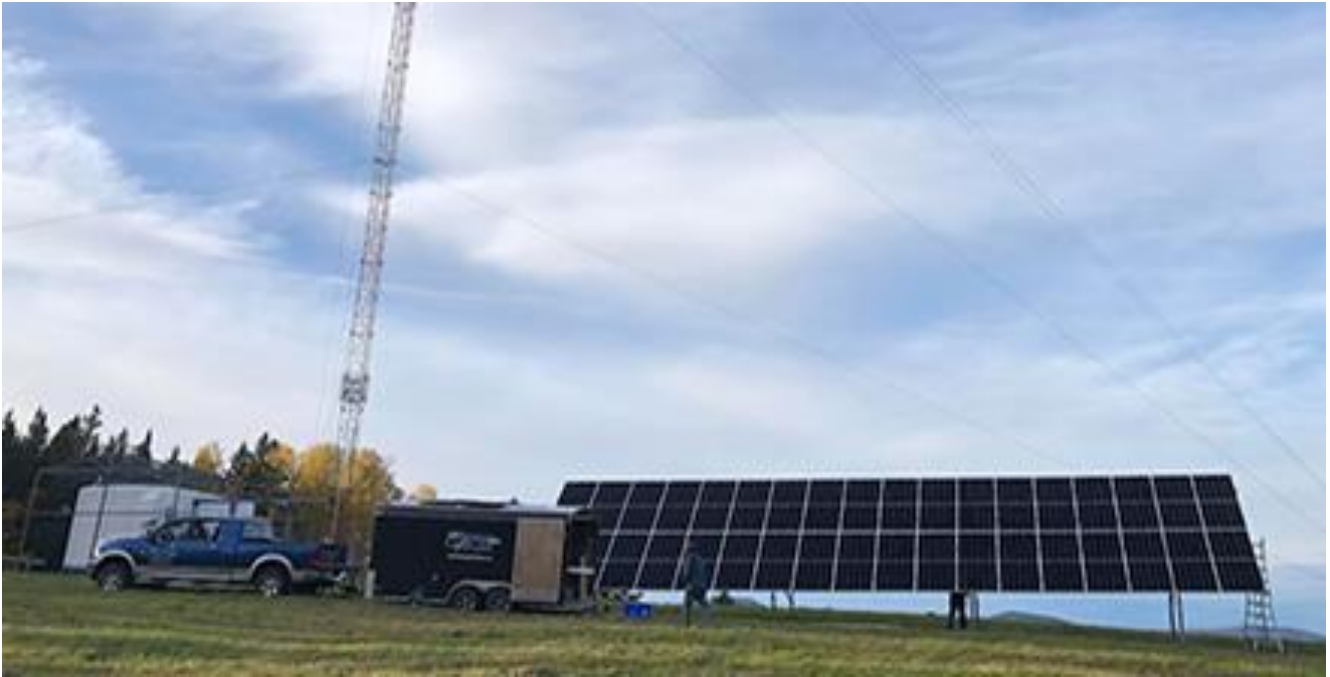
The solar panel located in Pointe La Nim, New Brunswick
